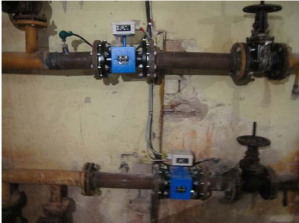
Meter for heating
