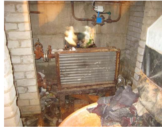
Meter for hot water
