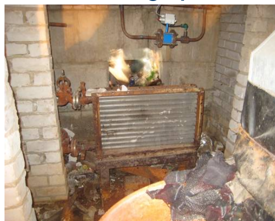
Meter for hot water
