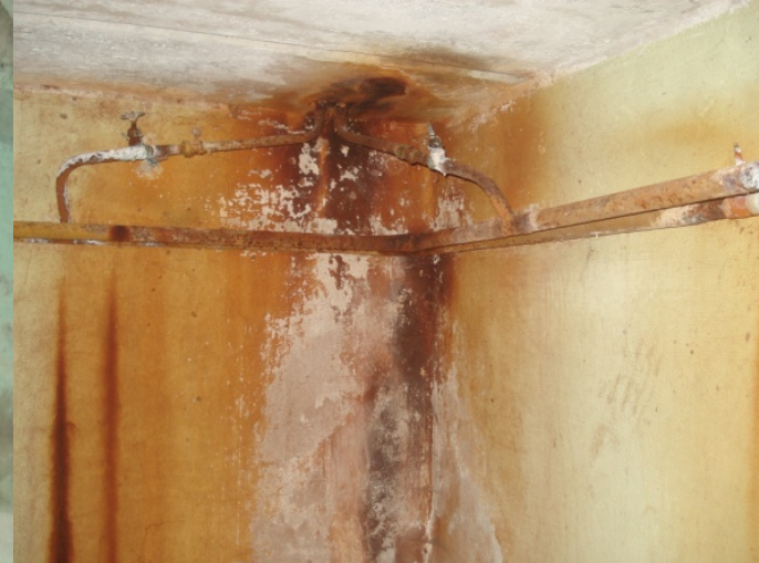
Central Heating pipes
