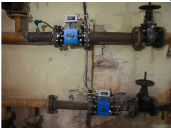
Meter for heating
