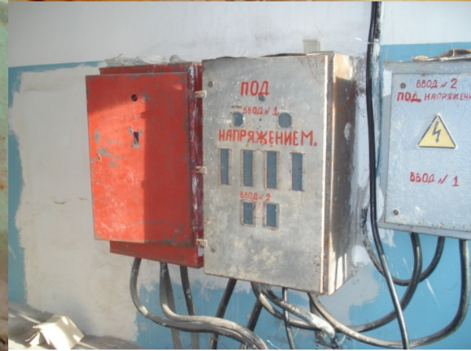
Electrical fuse box
