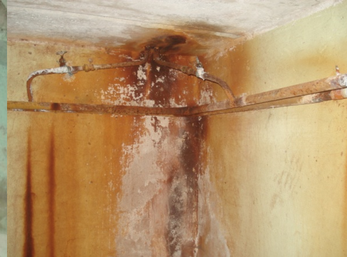
Central Heating pipes
