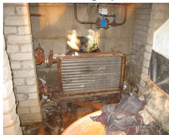
Meter for hot water
