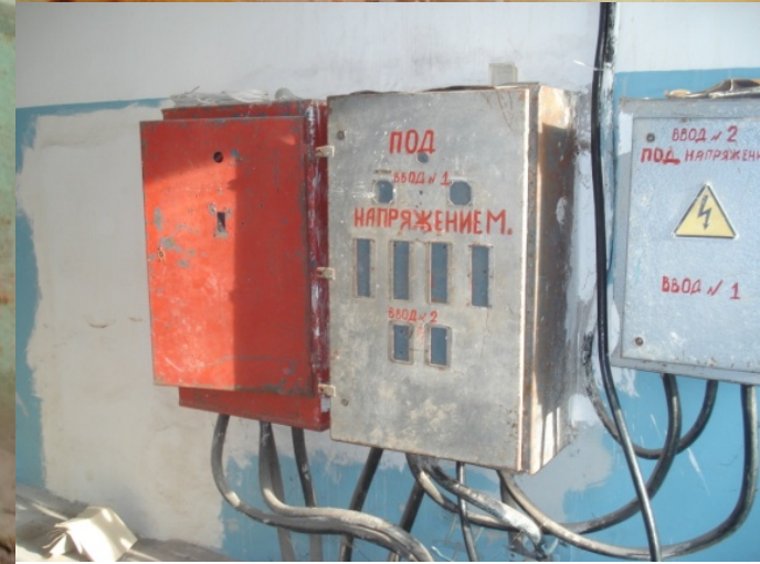
Electrical fuse box
